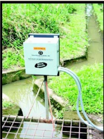
Sensor installed to monitor stormwater drainage ditch. Photo courtesy Occidental
