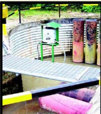
Detector installed above discharge retention area. Photo courtesy Occidental
